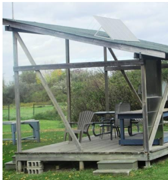
Solar panels mounted On the roof of the shelter.
